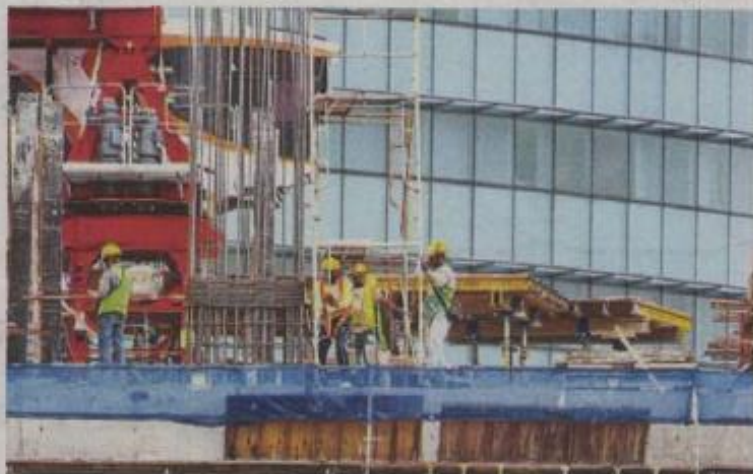
Key industry: A construction site in Kuala Lumpur. There are expectations that the sector could be a low-hanging opportunity for the government to pump-prime the economy.
