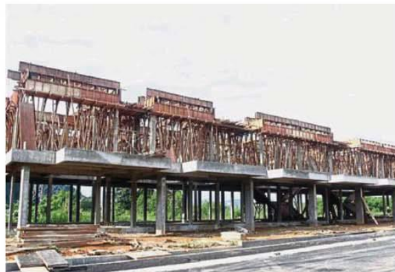
Several terrace houses being constructed at Taman Desa Bukit Perpaduan Hillville, Ulu Kinta.
